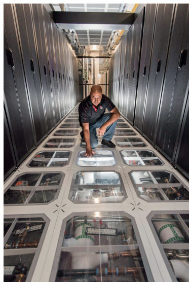
12. Cooling data center, saving water, by SandiaLabs
