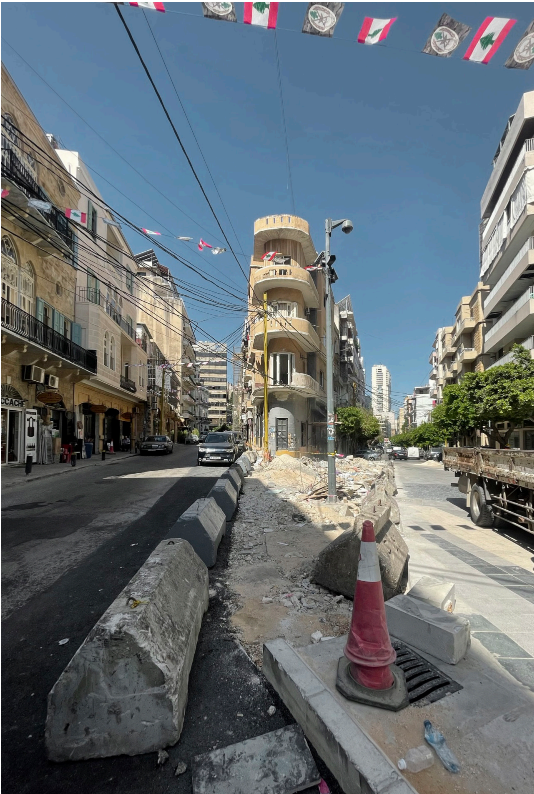
Figure 1 Site of the Failed Sidewalk, taken in July 2023, while construction works w on pause. The right side of the street is done while the left one is untouched, materials remain in the middle, awaiting a decision.
