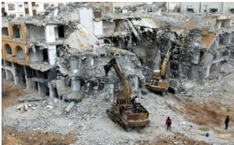
Figure 35: Demolition in Gaza after 2022 attacks
