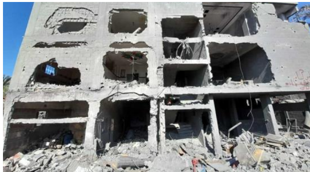
Figure 31: A building in Gaza struck by tank shells
