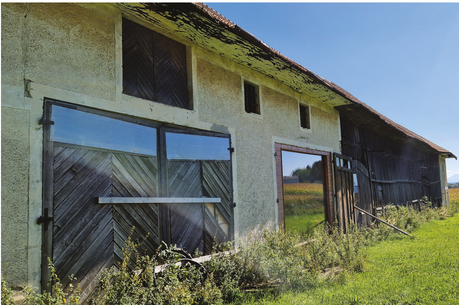
Figure 08.03 North-western external facade of "Leebgut" Vierkanterhof; (left to right) workshop doors, Herr S. Augl's new floor to ceiling window, and the light wooden structured, collapsing barn; underside of roof in bad condition (Ürmössy, 2023)
