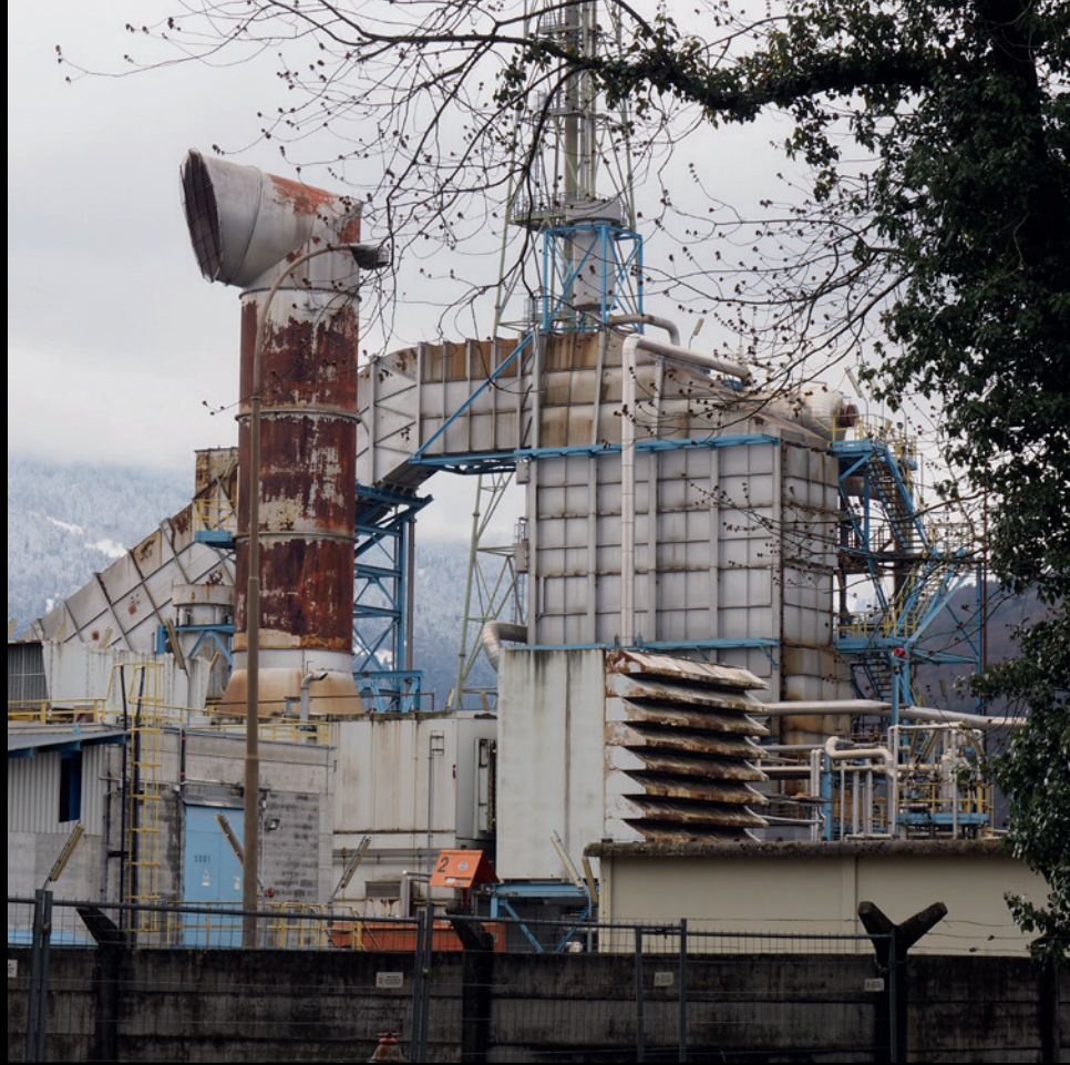
ventilation: metallic plates of various sizes
