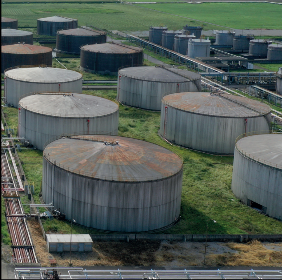
54 tanks - some thermally insulated
