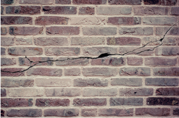
Figure 29. Photography of a damages brick wall
